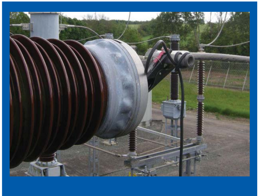
9. Clamps terminated by crocodiles supplied with BSG 1000, in action during a real test
