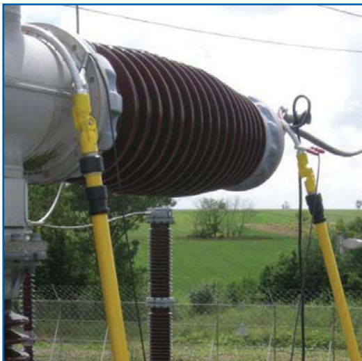
12. Arc clamp mounted on a real circuit breaker (with telescopic cranks)
