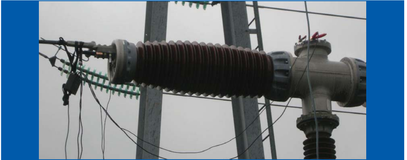
8. BSG remote head connection to a circuit breaker by crocodile clamps
