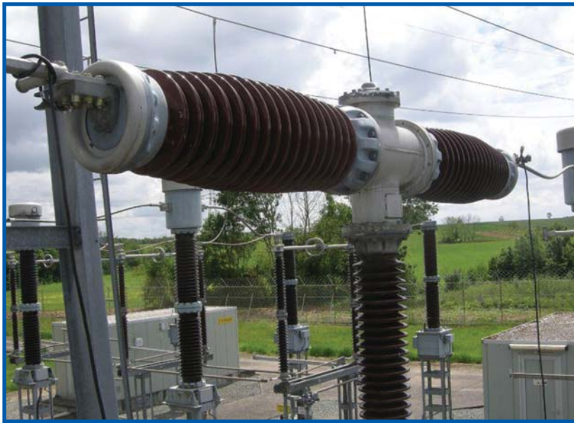
2. Two breaks per phase circuit breaker connected to ground on both sides
